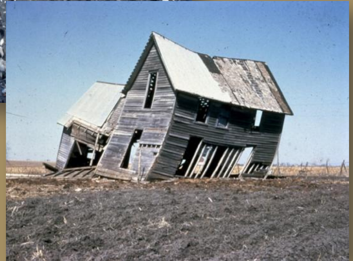
Collapsing house, NE
