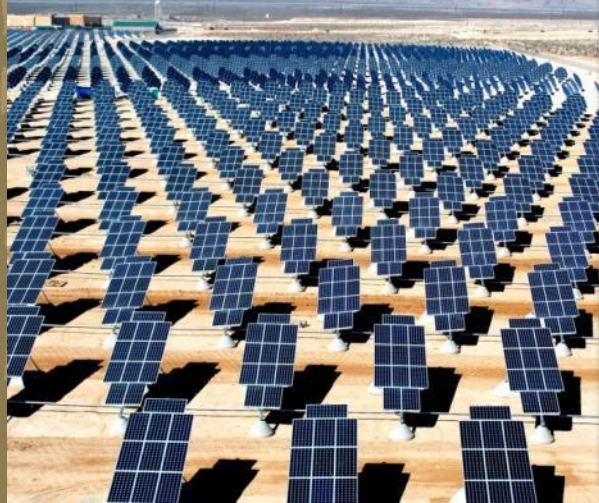
Photovoltaic array, Nevada
